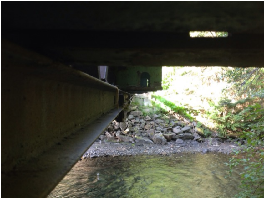
approx 20-30mm superstructure sag
