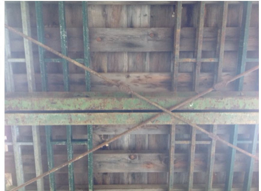
missing 10 foot section of steel stringer
