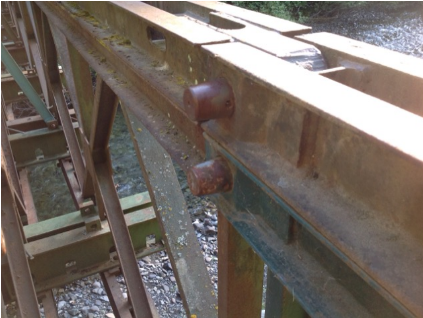
missing clips - approx 57 missing - all on top of the bay's
