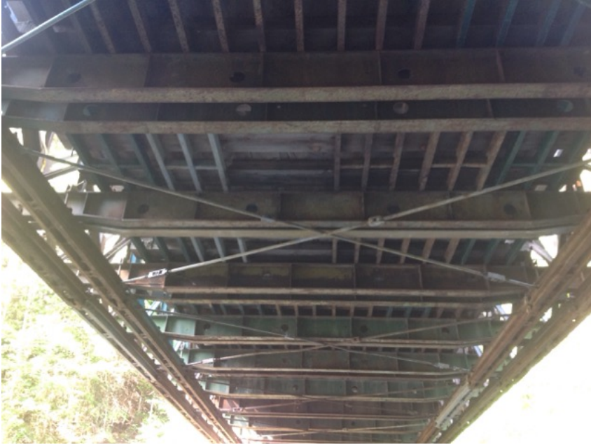
missing another 10 foot section of steel stringer
